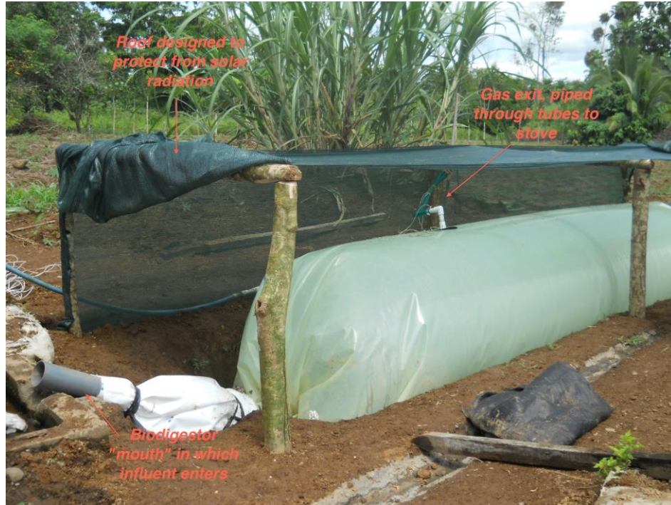
Figure 1: Taiwanese Biodigester in La Florita
